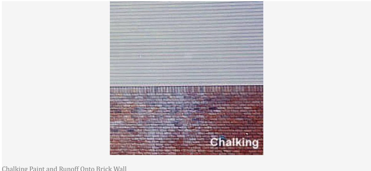
Chalking Paint and Runoff Onto Brick Wall
